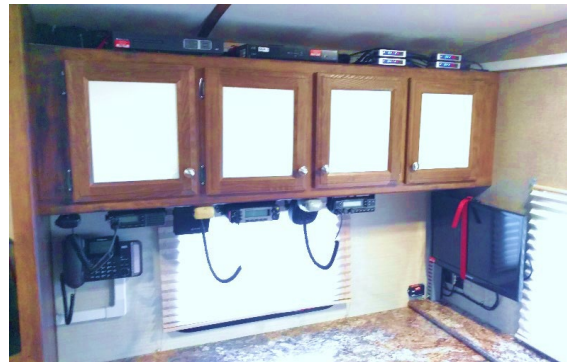
Communications Center in the MMU Trailer
